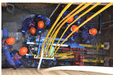
Restoration works with the use of horizontal drilling rig in the kahriz located in Aghdam district
